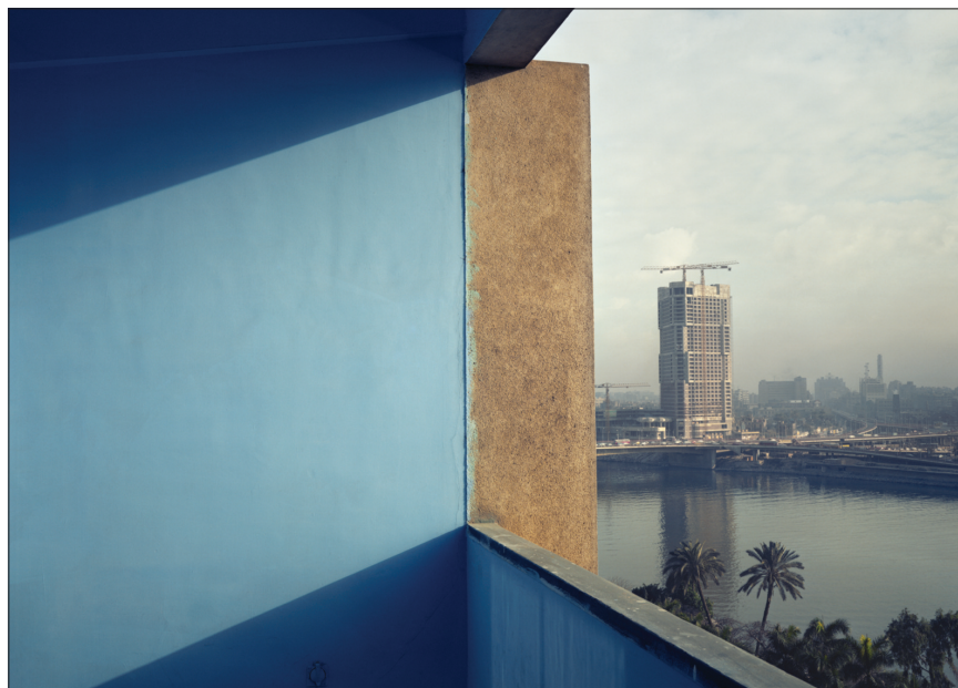
Adam Bartos, Cairo, Egypt (Ramses Hilton under construction) , 1980, pigment print, 31 \frac{1}{4} " x 41 \frac{1}{4} ". Gitterman.
